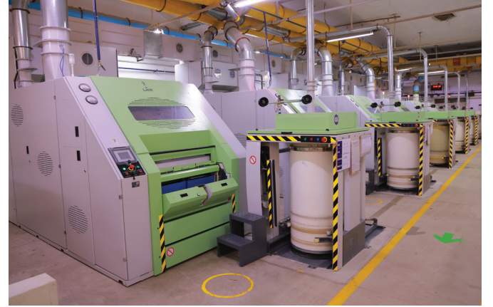
A view of new LMW Make Carding Machines installed at our Spinning Division.
