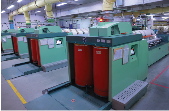
A view of new Rieter Make Comber Machines installed at our Spinning Division.
